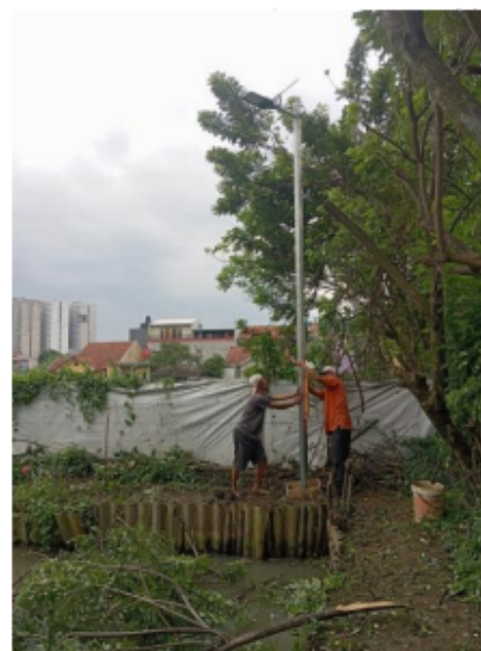
Gambar 7. Instalasi Lampu PJU Solar Cell (2)
