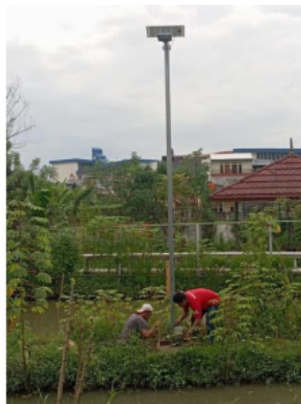
Gambar 6. Instalasi Lampu PJU Solar Cell (1)
