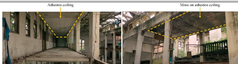
Figure 15. Asbestos ceiling on Warenhuis building
