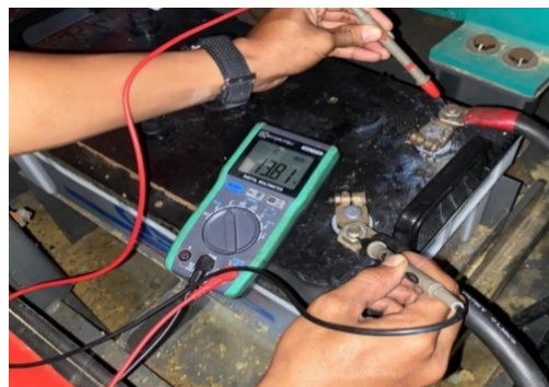
Figure 5 Measuring generator battery voltage using a digital multimeter
