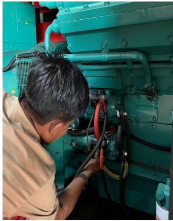
Figure 7 The old starter dynamo was still installed on the generator engine during the inspection.
