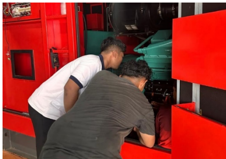
Figure 8 New starter dynamo as a replacement for the old starter dynamo
