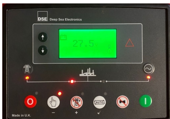
Figure 4 Battery voltage indicator on the generator control panel when the engine is running
